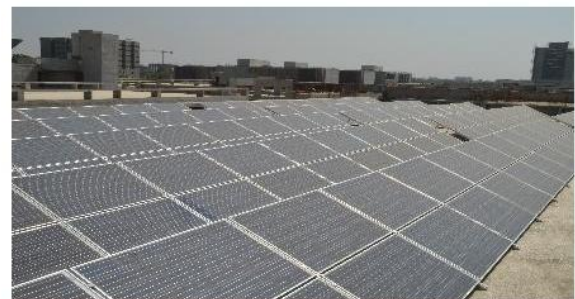
First Open University in India to have 50KV Solar Power Generation
